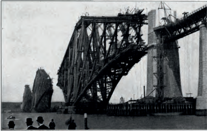
FIG. 228.—THE FORTH BRIDGE. LARGEST VIADUCT IN THE WORLD. FROM A PHOTOGRAPH WHEN IN PROCESS OF CONSTRUCTION. LENGTH, 8,290 FEET; HEIGHT ABOVE WATER, 361 FEET; MAIN SPANS, 1,710 FEET LONG, 150 FEET HIGH.
