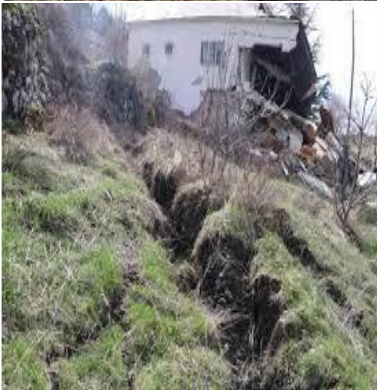
Fig. 4. February 6 earthquake ruptures in agricultural areas (Anonymous., 2023)
